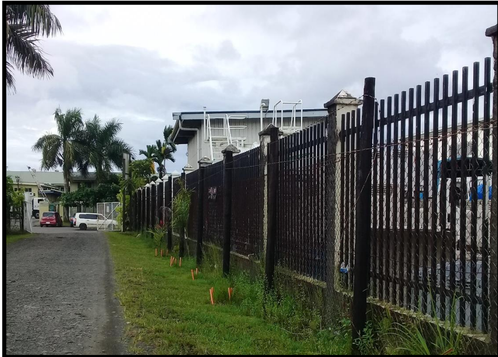
Fig1. Existing fence that needs to be changed completely
