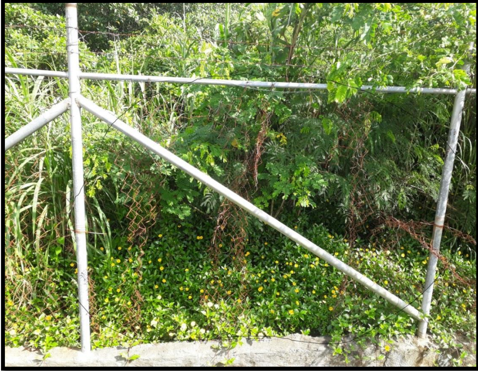
Fig1. Section of fence where chain link & barbed wire is missing
