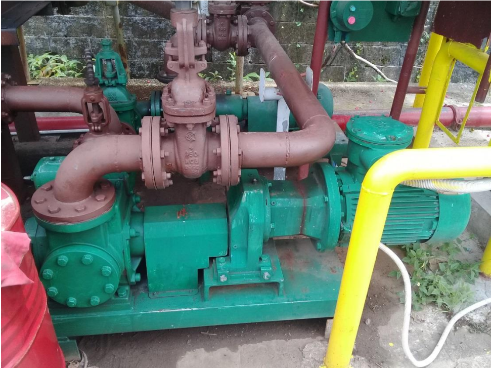
Fig1. Existing pump unit at Kinoya Power Station
