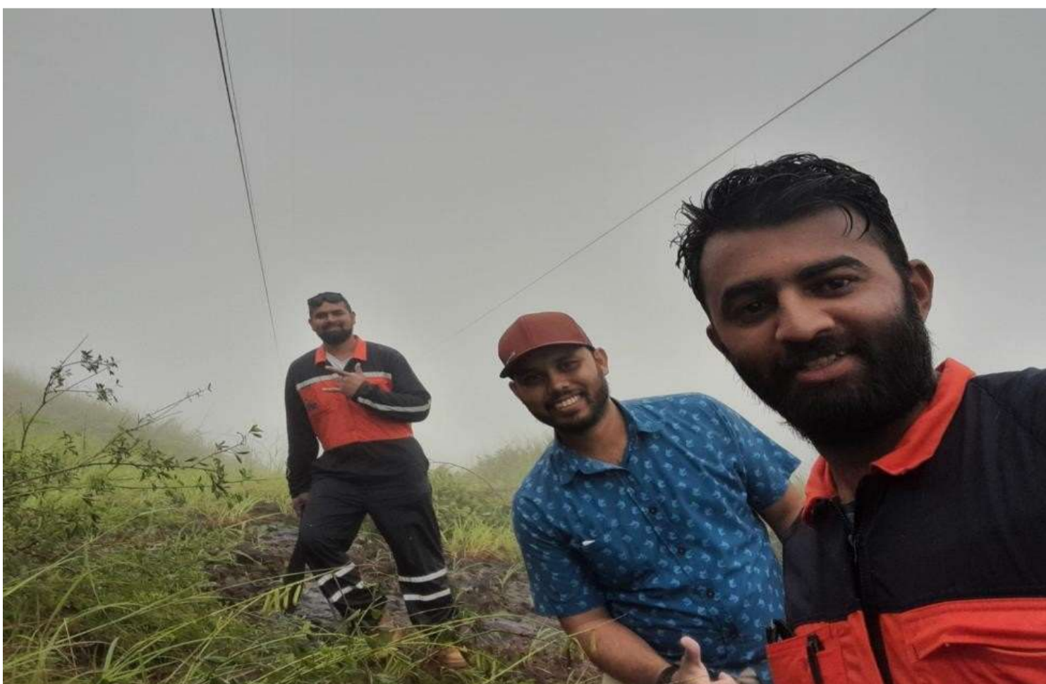
The EFL team returning after removing a fallen tree from the 132.00volts Vuda to Nadarivatu Transmission line around 6pm thisafternoon, Wednesday 12 th January 2022. Left to right: Shivneel Singh, Amitesh Chandra & Vinaal Prakash
