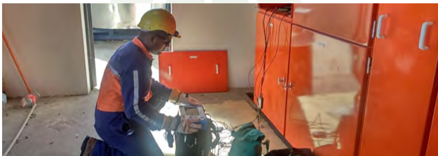
FEA Metering Technician carrying out metering system re-calibration work at Punjas Biscuit factory in Lautoka. This is to ensure that the customer's meters are functioning properly and recording correct consumption.
