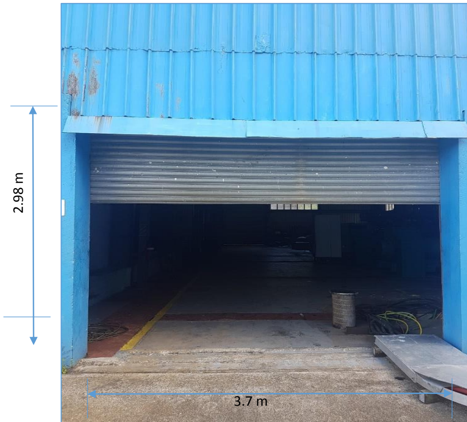
Figure 2 shows the view of the front end shutters of the Deuba Power Station with the measurements in meters.
