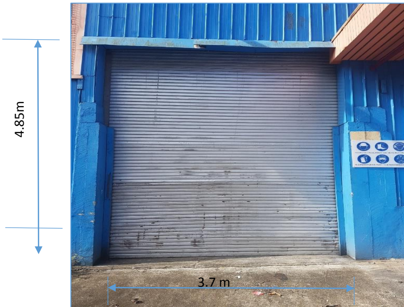
Figure 1 shows the view of the rear end shutters of the Deuba Power Station with the measurements in meters.
