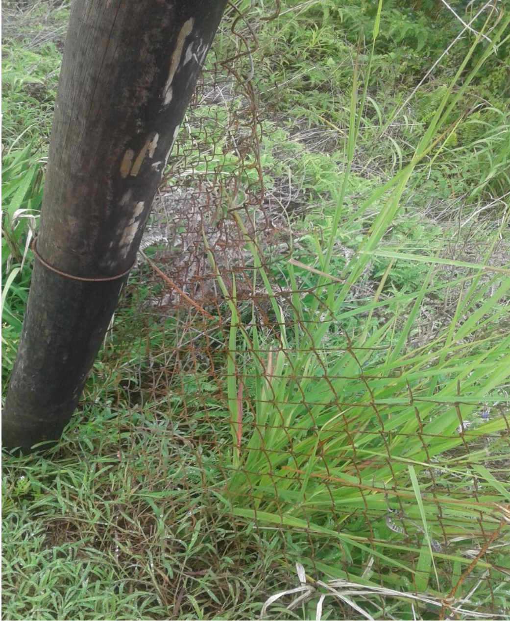
Fig 2. Section of fence where chain link is damaged
