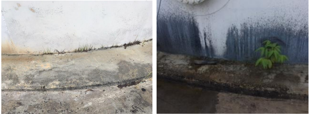
Figure 2 and 3 shows the cracks at the base of the fuel tank which leads to growth of grass and plants
