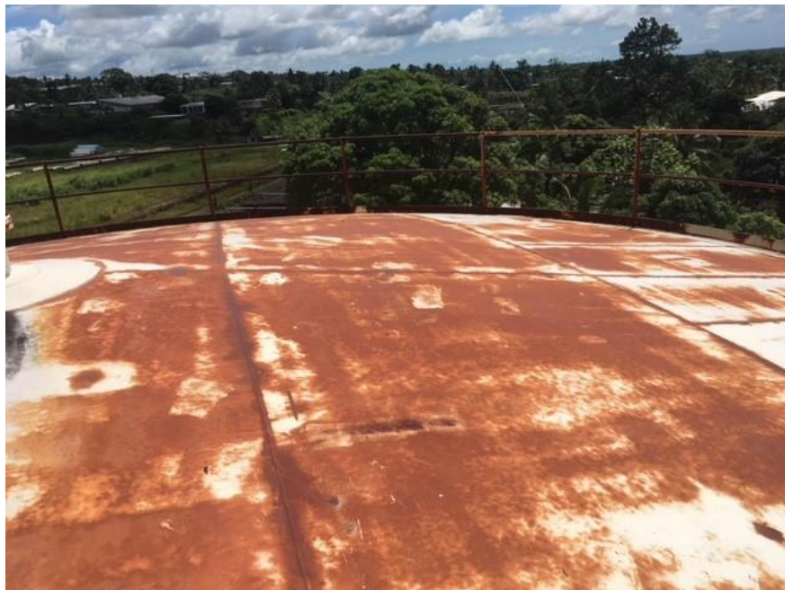
Figure 4 shows the top surface of the Fuel Tank.
