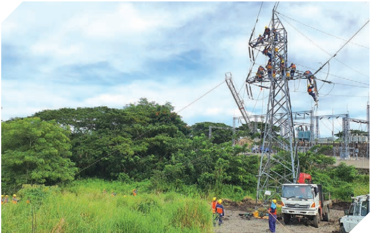
EFL Transmission Team carrying out maintenance on the 132kV Transmission Tower near Vuda Substation.
