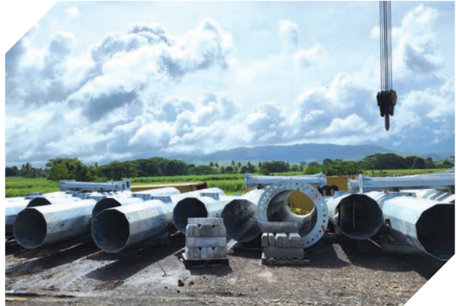
EFL received steel monopoles and lattice towers for the new 132kV Virara to Koronubu Network project.
