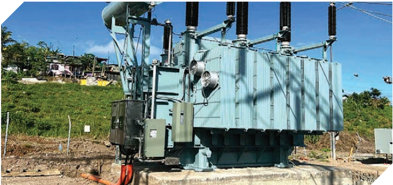
Installation of the new 132kV/33kV T2A Power Transformer at Cunningham Road Switch Yard.
