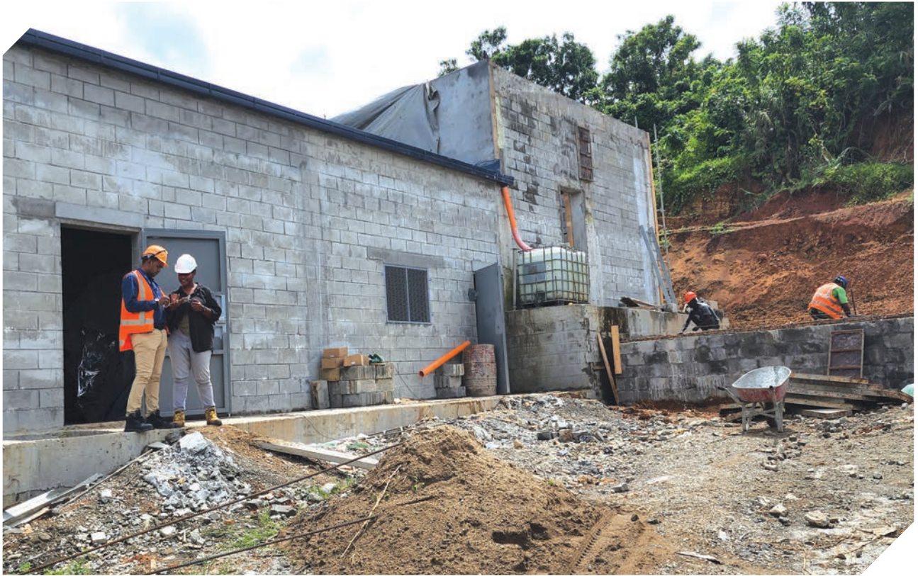
Waitolu 33kV/11kV zone substation under construction and expected to be completed in 2023. This substation will be part of the Viria water reticulation project.
