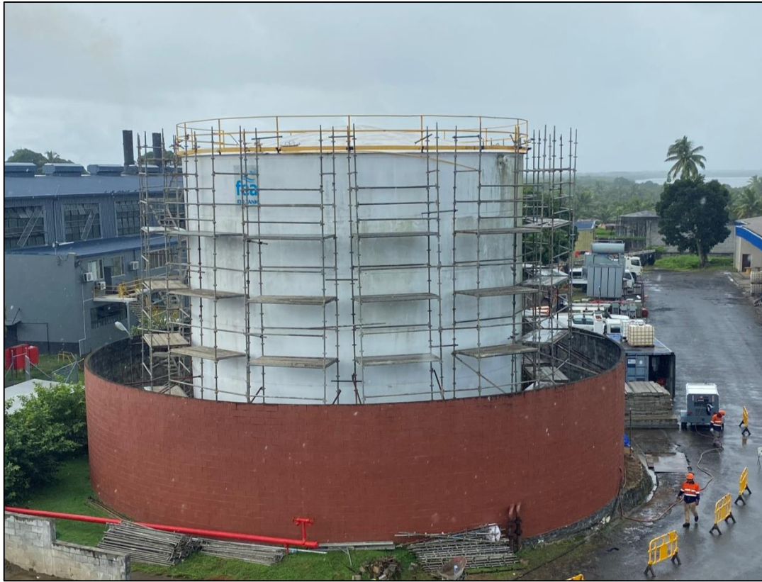
Figure 1: IDO Bunker Tank T1 at EFL Kinoya Power Station
