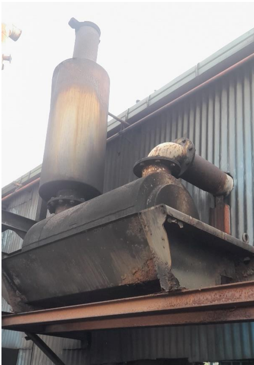
Figure 1: Existing horizontal and vertical silencer on site
