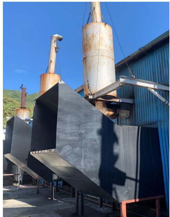
Figure 2: Existing radiator vent on site
