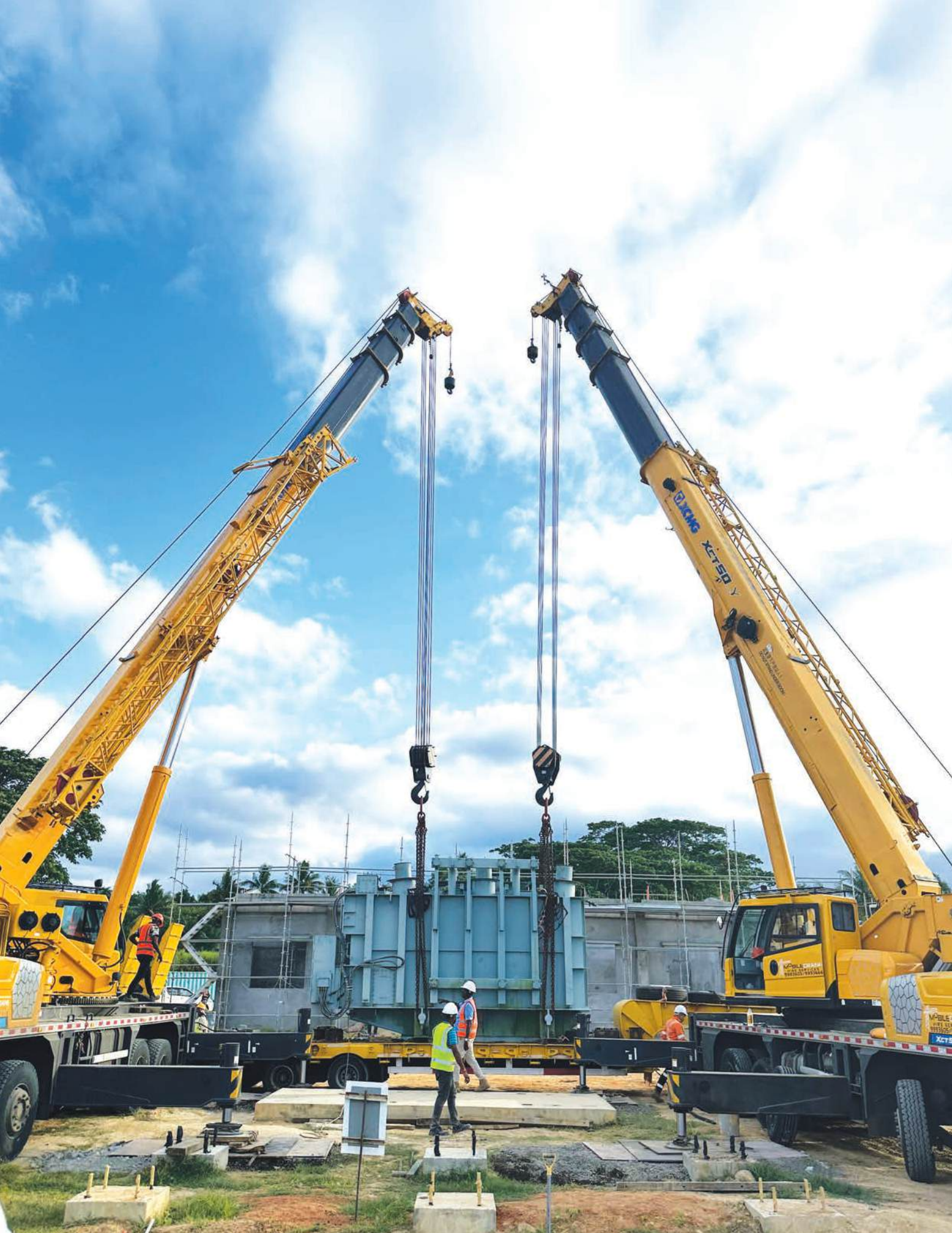
Installation of 132/33Kv Transformer on Pad at Koronubu for Virara to Koronubu, Ba 132kV Transmission Line Project.
